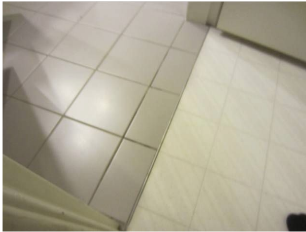
Cracked grout noted to bathroom floor tiles.
