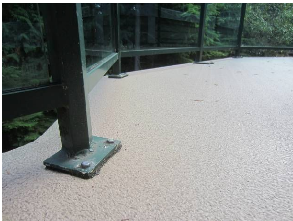
Recommend sealing around balcony railing penetrations.
