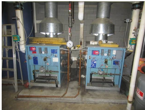
Hot water boilers.
